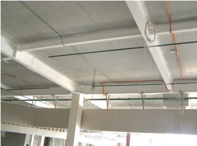
Fig. 1. View of a steel-reinforced concrete floor fragment
